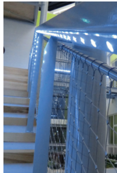
Lighting of the handrail by LEDs
